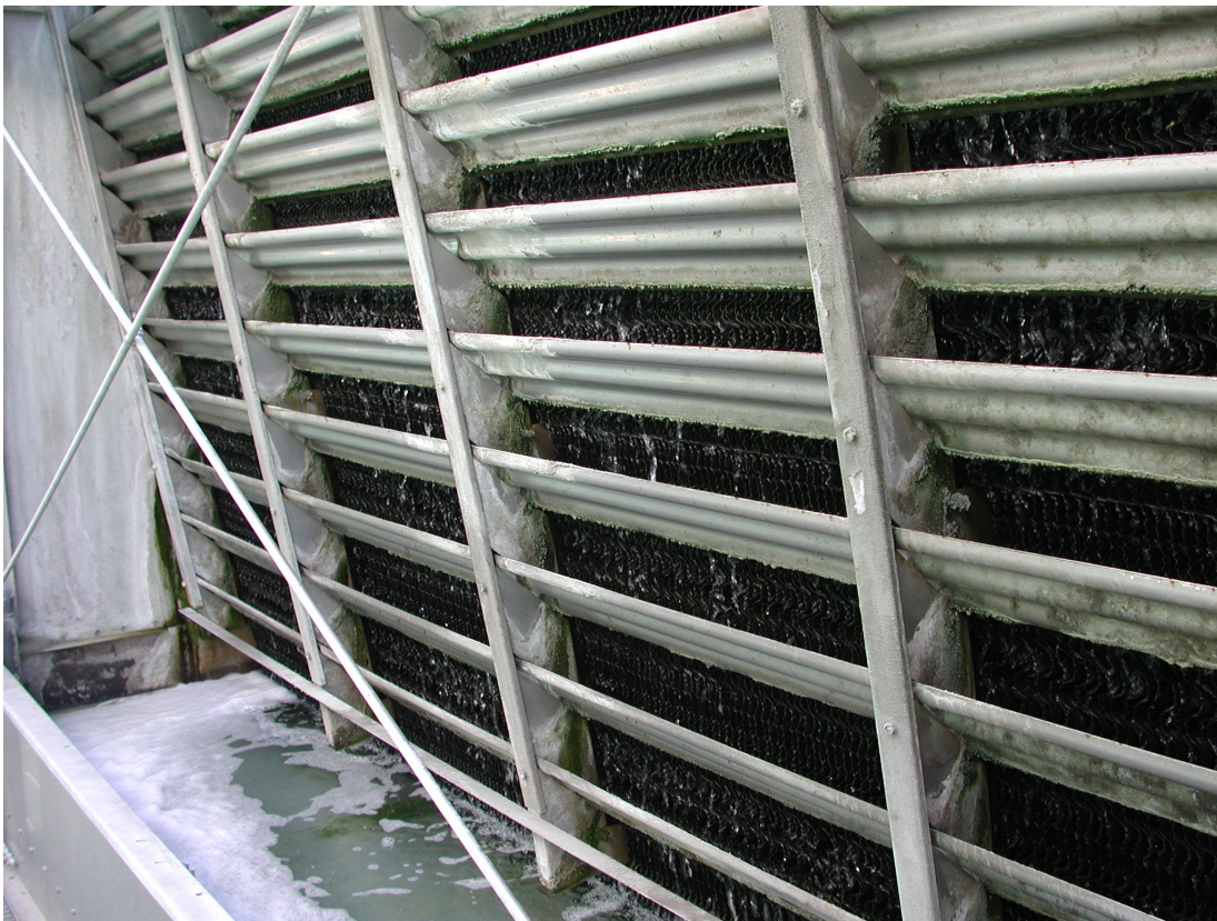
Fig 2: Clean cooling water systems operating at high pH using chlorine.
